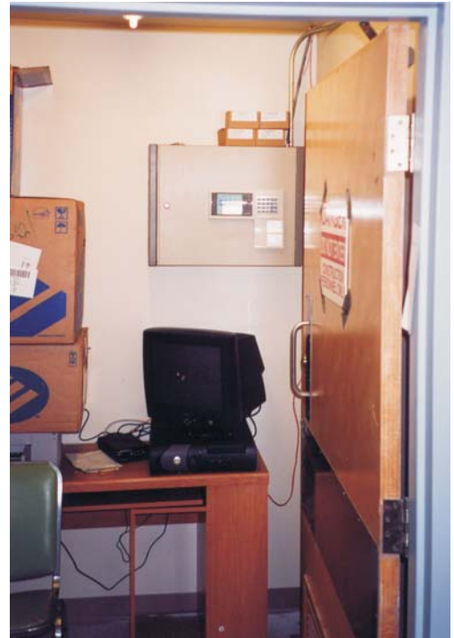
All units are controlled from a MJ-103MTRA central controller.
