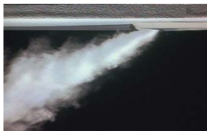
The unique airflow pattern ensures that ceiling tiles do not smudge.
